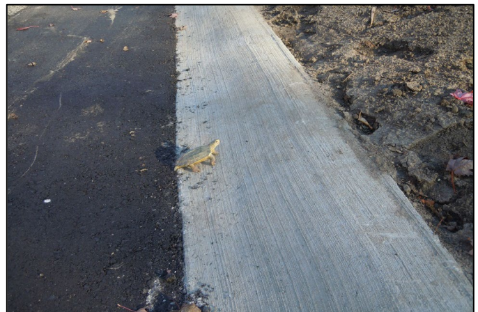
Figure 1. Sloped curb installed at a site in Ottawa. Toy turtle (8 cm carapace length) for scale.
